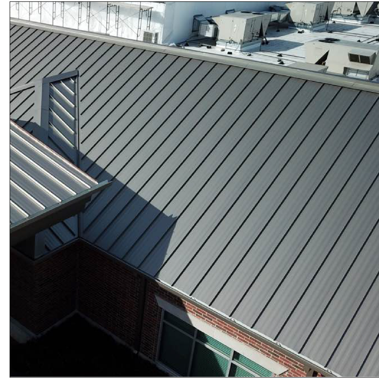
2 STANDING SEAM METAL ROOF BY: ASC BUILDING PRODUCTS COLOR: SLATE GREY/ DESIGN SPAN HP
